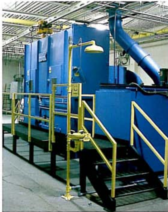
A typical stripping system includes the solution tank and a rinse tank.
